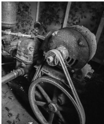
Pump in the Budd pump house (photo Jim Caffrey)
